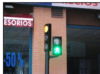
Traffic lights with LED lamps at a pedestrian crossing
